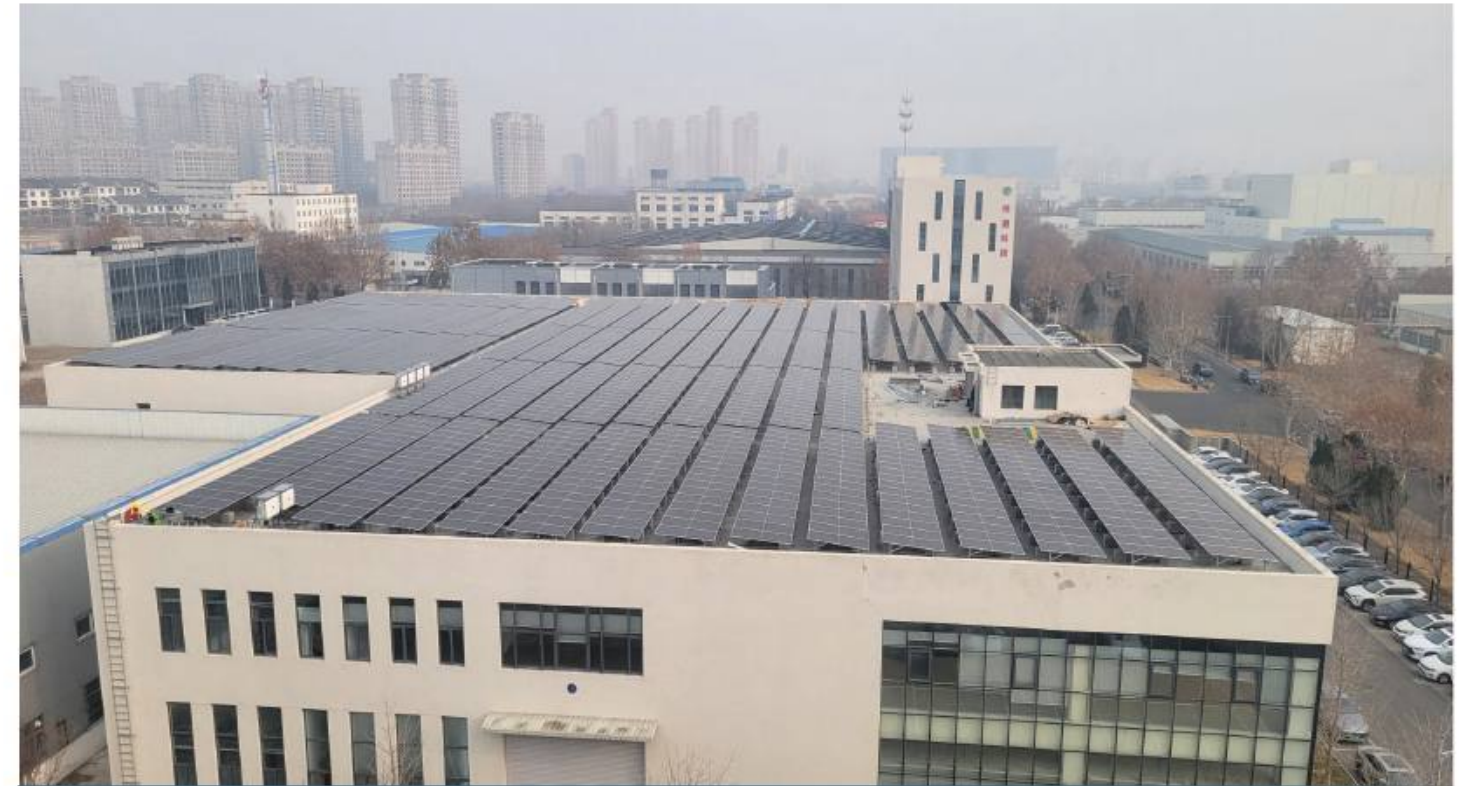
Tianjin - Ruineng Electric Industrial Park BIPV Project (Rooftop)
