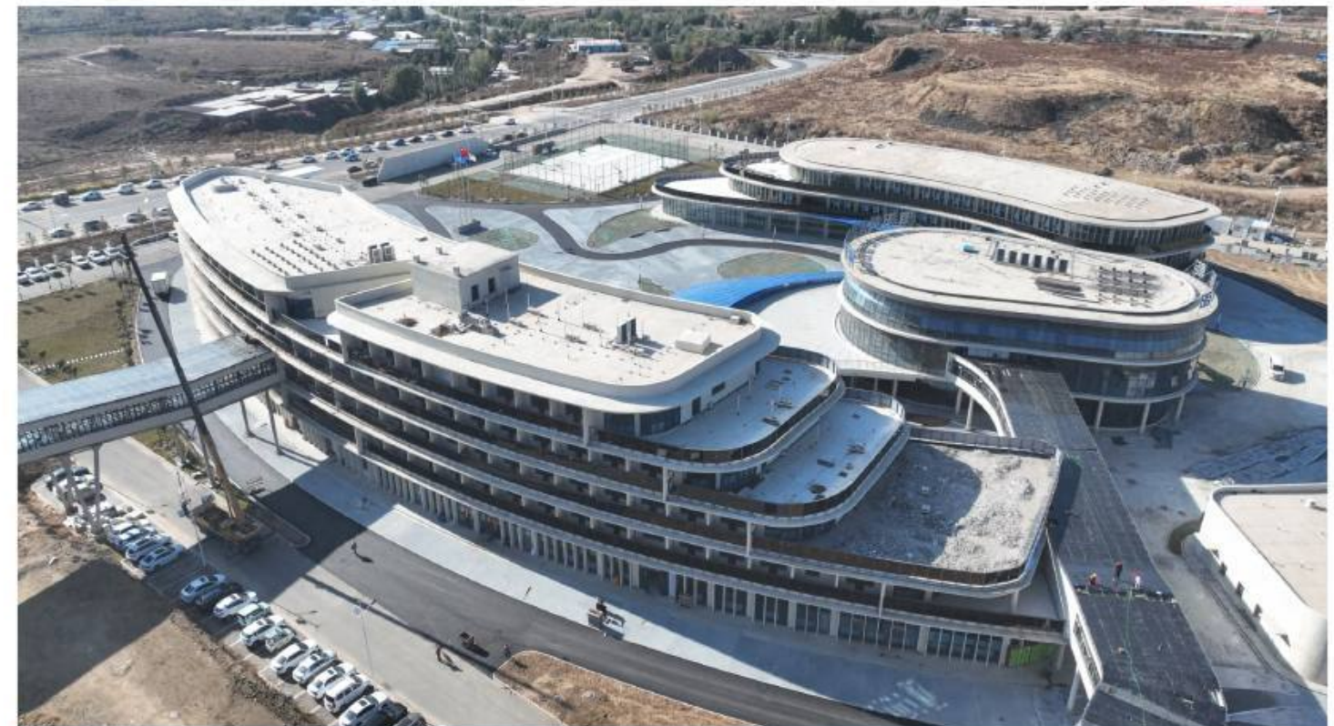
Baotou - Northern Smart Energy Building BIPV Project (Skylight + Railing)
